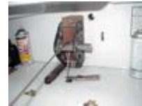
Center Board Cable
