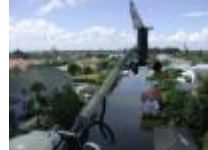
Wind Vane Repair
